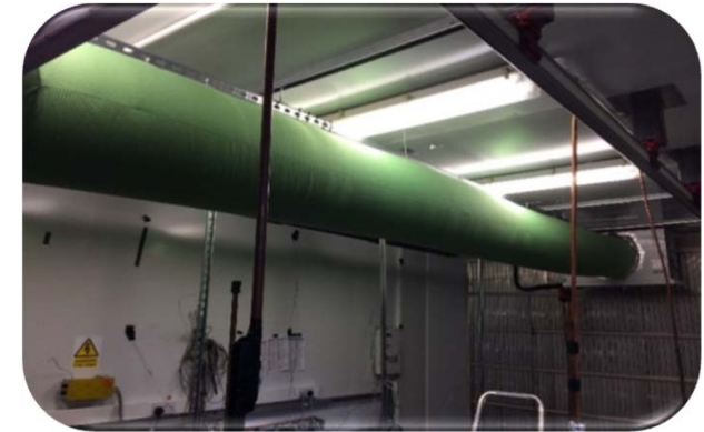
Test facility, reference case.
