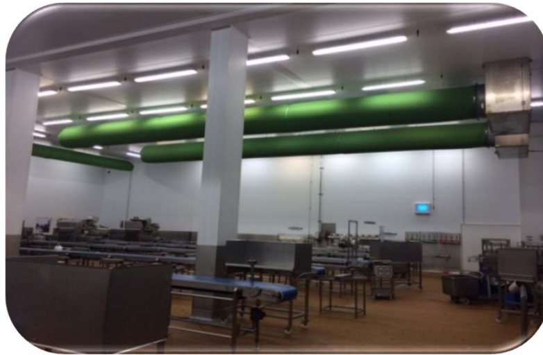
Air distribution via fabric ducts
